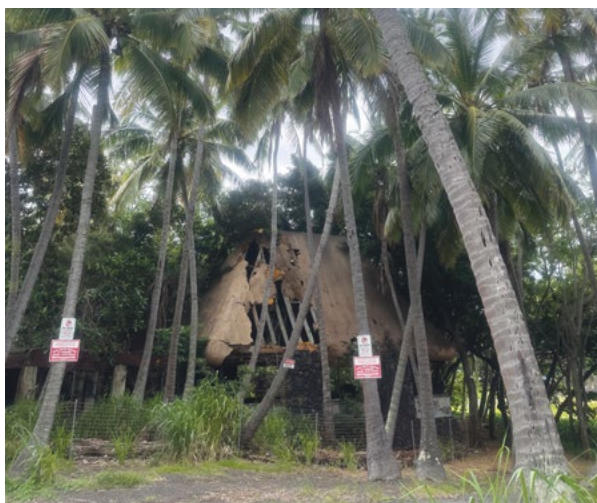
The collapsing A-frame of the Punalu'u Village Restaurant from the 1970s sits overgrown and neglected on private parcels ma uka of the beach. When Hawai'i's sugar industry began to collapse in the 1970s, landowners shifted focus to resort and tourism ventures.
