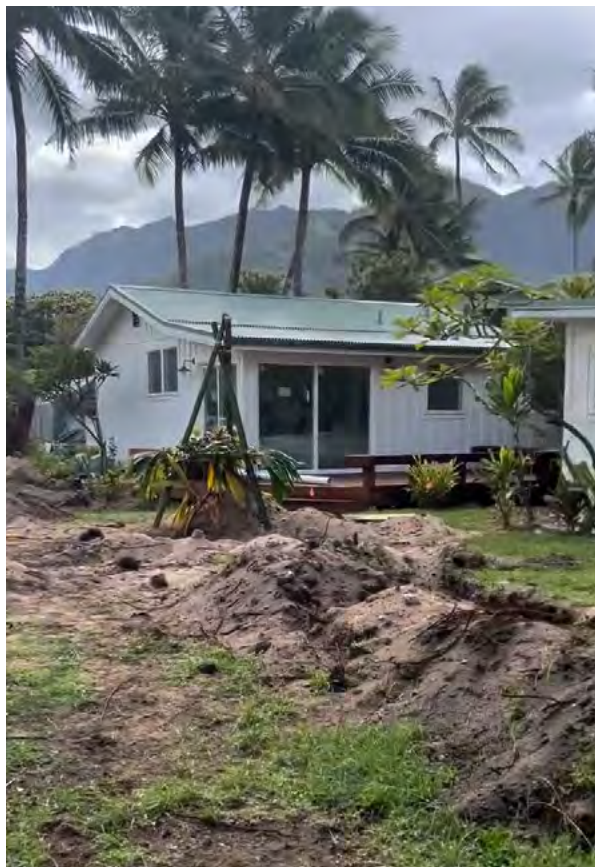
For now, installation of new septic tank and leach field at a residence in Wainiha, Kaua'i, has been halted due to the discovery of iwi kūpuna until state and county agencies determine next steps. - Photo: Megan Wong
