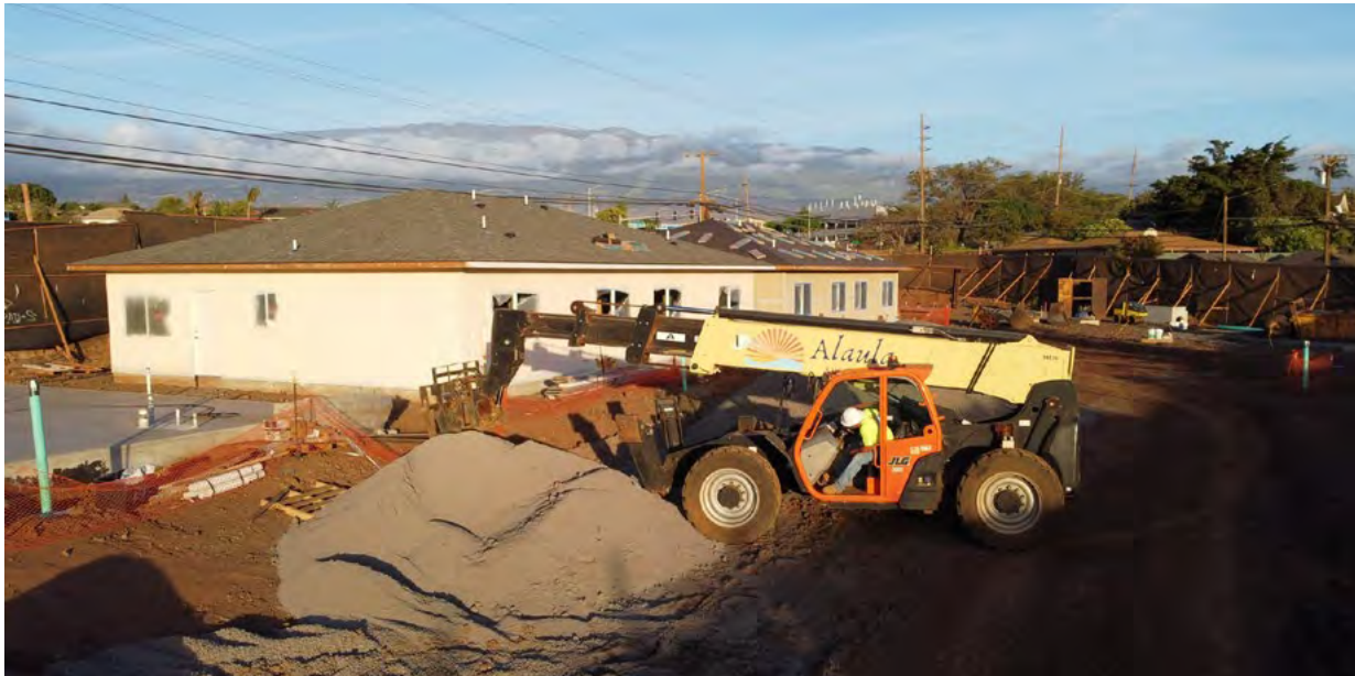
Hale Kaiola in Kihei, currently under construction by Alaula Builders, is a priority project identified in the Maui Housing Plan. The project will provide 40 new affordable duplex homes for Maui residents. For more info go to: www.Alaula.org . - Photo: Alaula Builders
