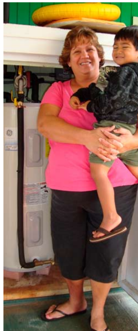
Hawaiian homestead resident Iwalani Martin of Anahola, Kaua'i, holds her grandson Sammy Kauvaka in front of her family's new solar hot water system, paid for with federal stimulus funds. - Photo: Courtesy of the Council for Native Hawaiian Advancement
