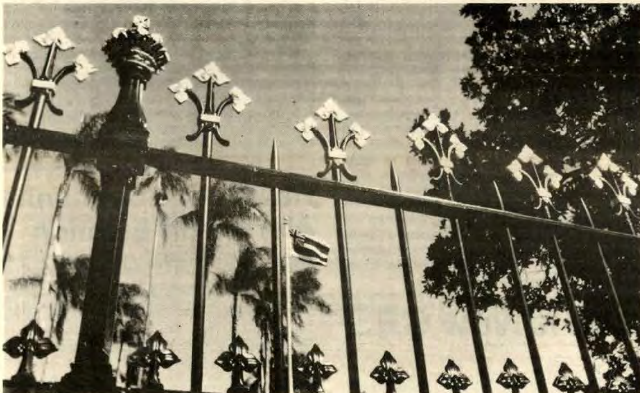
The restored Royal Mausoleum fence is decorated with 350 flower motif finials and 50 small crowns. The finials are a decorative element thought to have a religious connotation, and the crowns may be patterned after the crowns of the Hawaiian alii, complete with taro leaf replica. The fence was ordered to specification from the prestigious Coalbrookdale Co. in England by Kamehameha IV.—Photo by Bruce G. Lum, Kamehameha Schools/Bishop Estate.
